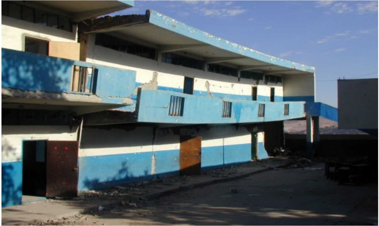
Fig.6 School building in Moquega. Partial collapse due to short column failure
